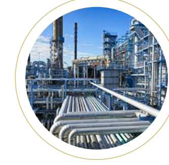
INDUSTRIAL HIGH-PRESSURE MAINS
