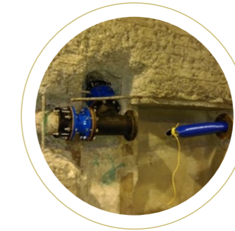
FIRE WATER MAINS
