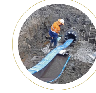
SEWER RISING MAINS
